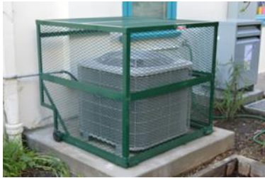
New HVAC systems provide fresh ventilated air, more efficient heat in the winter and cooling in the summer
