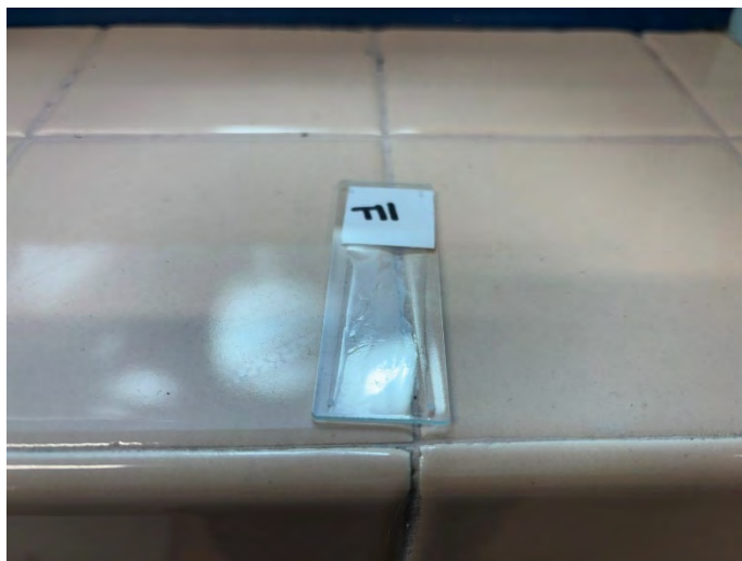
Photo #78: Building H – Girls restroom – Wall – T-11
