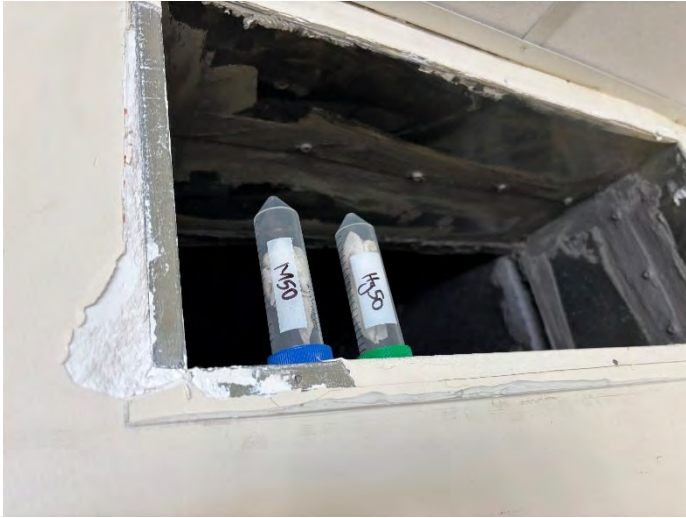
Photo #97: Classroom 11 HVAC Vent – M/Hg-50
