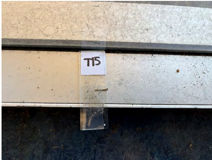
Photo #85: Building O – Cafeteria – Windowsill – T-15
