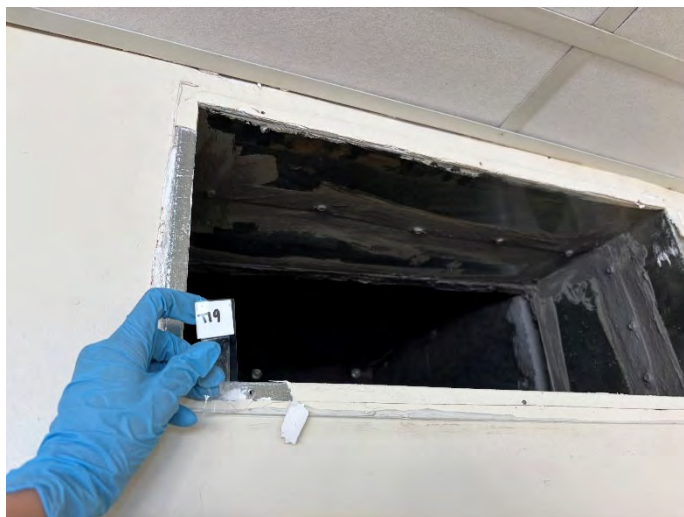
Photo #94: Building B – Room 11 – HVAC – T-19
