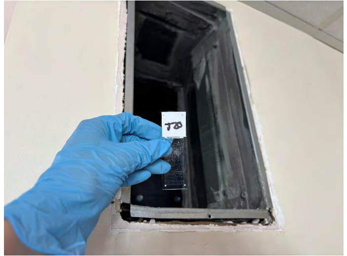
Photo #98: Building A – Room 20 – HVAC – T-20
