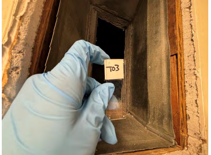
Photo #22: Building A – Room 17 – HVAC – T03
