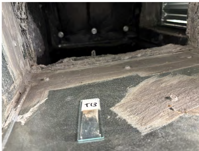
Photo #80: Building H – Room 3 – HVAC – T-13
