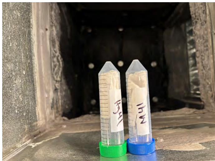
Photo #81: Classroom 3 HVAC Vent – M/Hg-41
