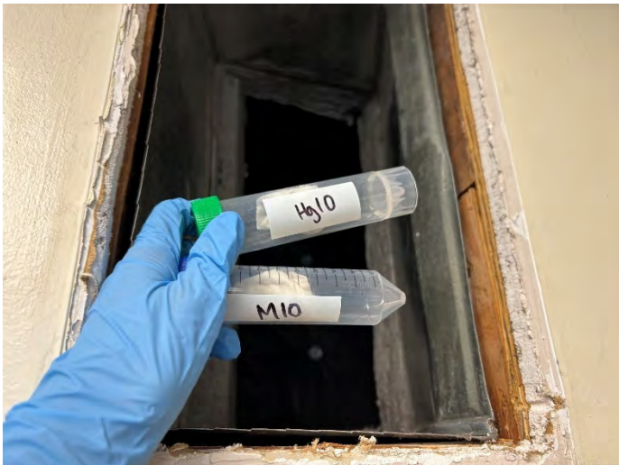
Photo #23: Building A – Room 17 – Supply HVAC – M/Hg-10
